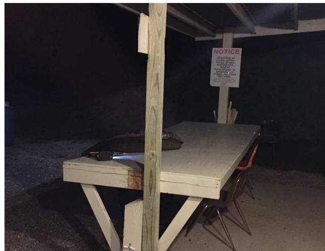
The member immediately reported the incident to me and with the help of Adam Leonberger we were able to repair the broken pole that evening before any wind could cause more damage. It happens.
